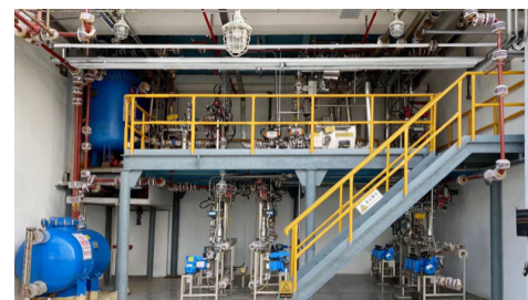
Corning AFR G5 industrial Installation
