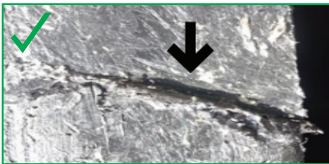
Non-extensive, superficial damage to the edge or sides of the flange no greater than 1 inch
