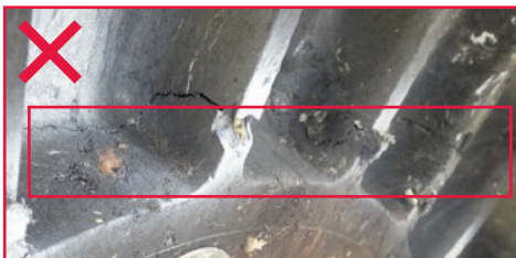
Large (greater than 1/16 inch) cracks in side or edge of flange
