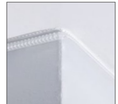
Clear Track Hallway Fibre Pathway
