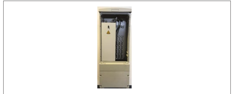
GF-NVT in KVZ92
